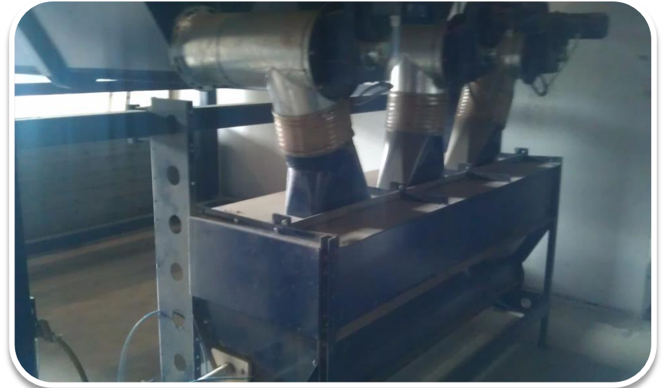
Crusher in operation
