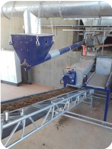
Back-mix unit, HK mixer and conveyor belt to Pollo dryer
