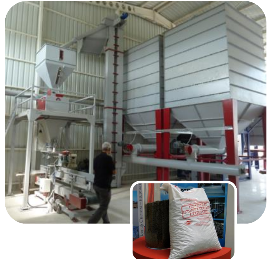
25 kg bag filled by the bagging station
